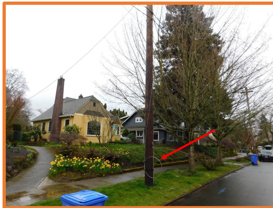
Inadequate guy installation
