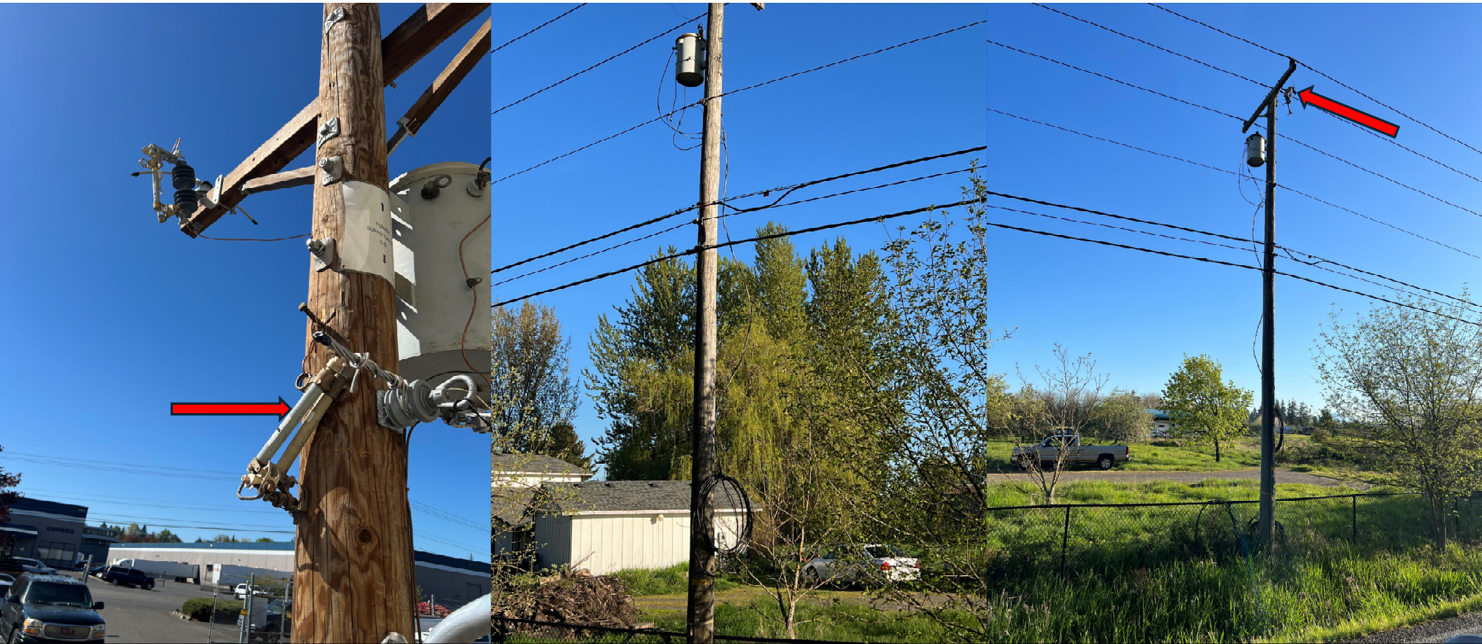
Abandoned Equipment in the Supply Space
